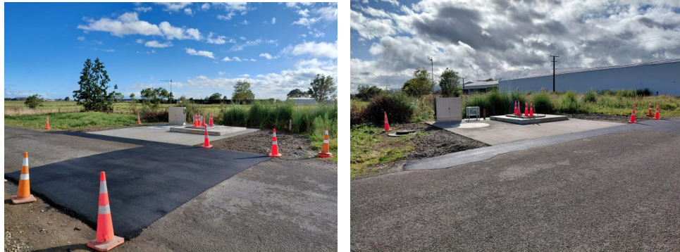
New Bryce Street pump station
