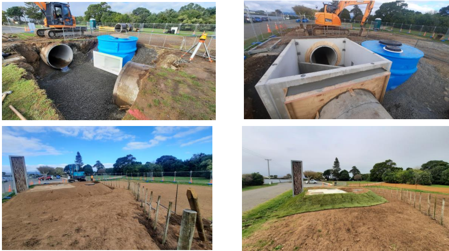
The images above provide an overview of the Queen Street Stormwater Intervention Device project in Levin from installation to reinstatement.
