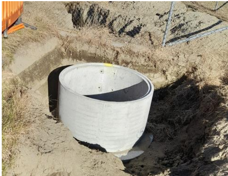
Leachate pump riser
